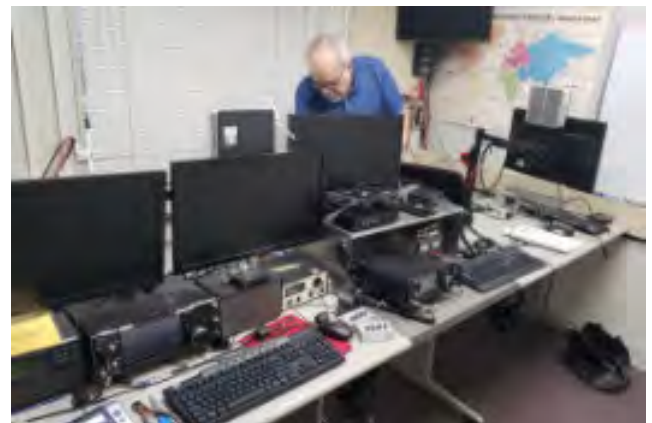
Steve VE7SXM in process of cable reorganization and conversion to 100% 12v battery power, including addition of inverter and transfer switch.
