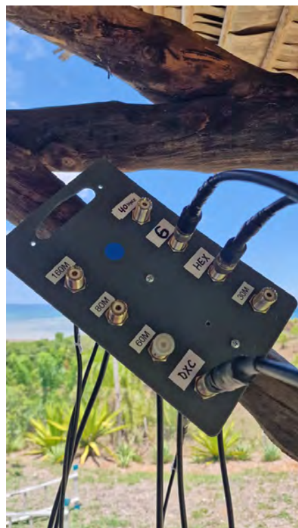
Coax patch panel
