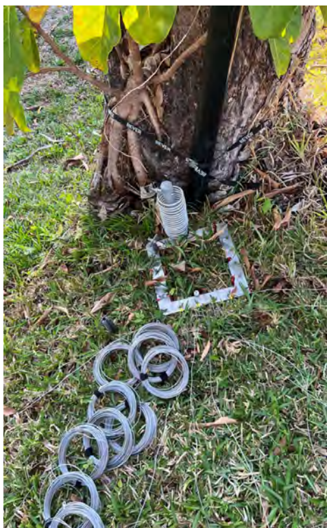
160m vertical matching unit and radials
